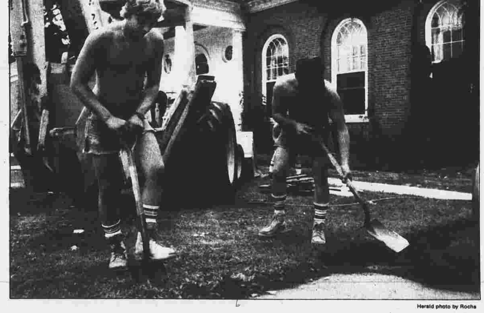
Laying the groundwork Paul Muszynski, left, and Jim Salvatore, both of East Hartford, get the grounds of the Mary Cheney Library ready for repairing and replacing the cement sidewalks. The work, being done by S. Aleria & Sons Contractors of East Hartford, started Wednesday and is scheduled to be finished by Friday. The library will remain open during the work.
